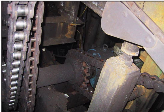
Scale, oxide and rust creates excessive wear to the chain.
